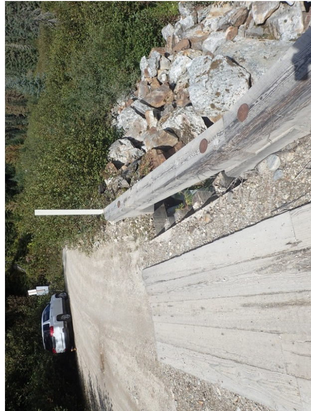
Figure 12: Right approach - note gap between decking and rail.
