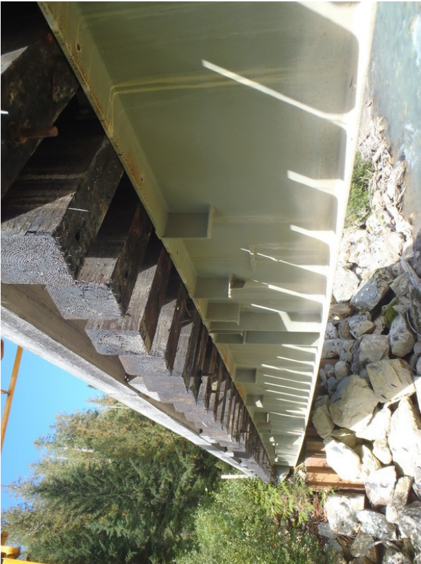
Figure 14: Exterior girder & tie condition, girder 4 shown.
