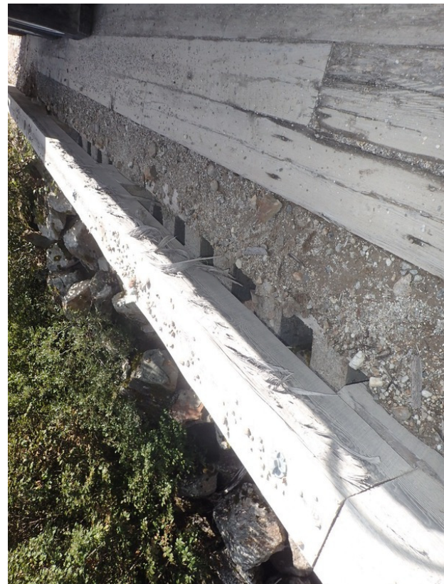
Figure 11: Minor rub damage to rail.
