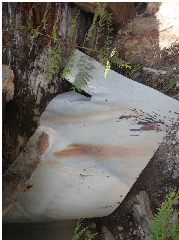
Figure 24: Right abutment upstream face - typical condition of flashing.
