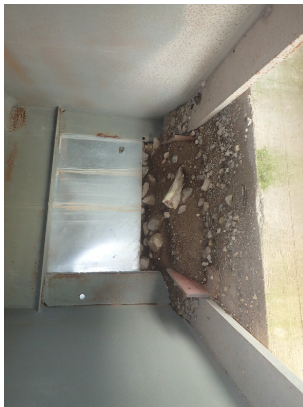
Figure 23: Right abutment - typical condition of flashing between girders and debris collecting on bearings.
