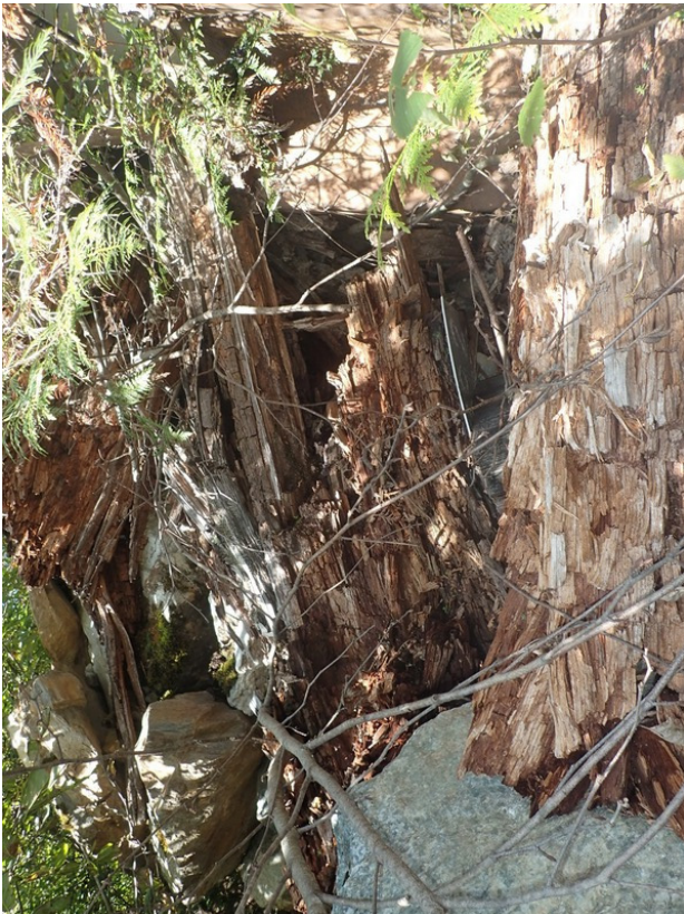
Figure 25: Right abutment downstream face - disintegrating ballast logs.
