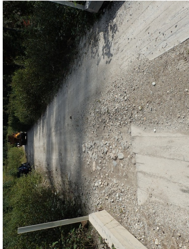
Figure 8: Left approach - note potholes at end of deck.
