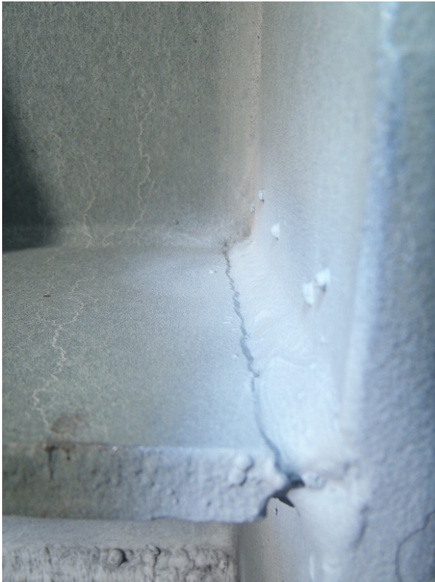
Figure 18: Typical undercutting on stiffener weld - girder 4 location C downstream stiffener shown.
