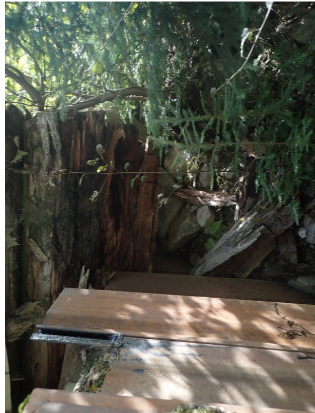
Figure 27: Left abutment downstream face - disintegrating ballast logs.
