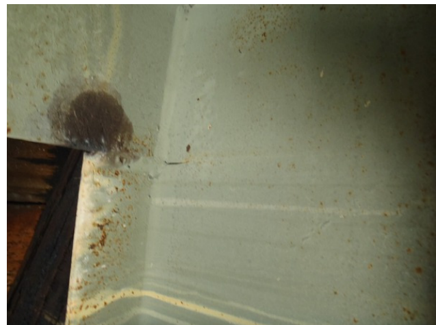
Figure 19: Torch cut in bay 2 diaphragm adjacent to right abutment.
