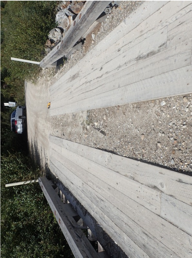
Figure 10: Typical deck condition.
