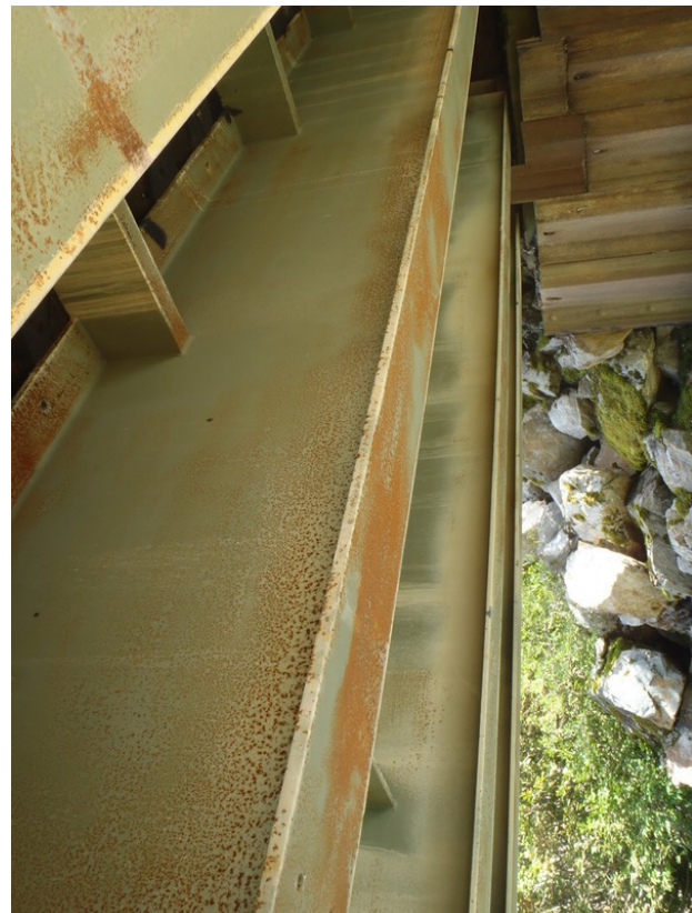
Figure 15: Interior girder condition, girder 3 shown - coating failure with light corrosion.
